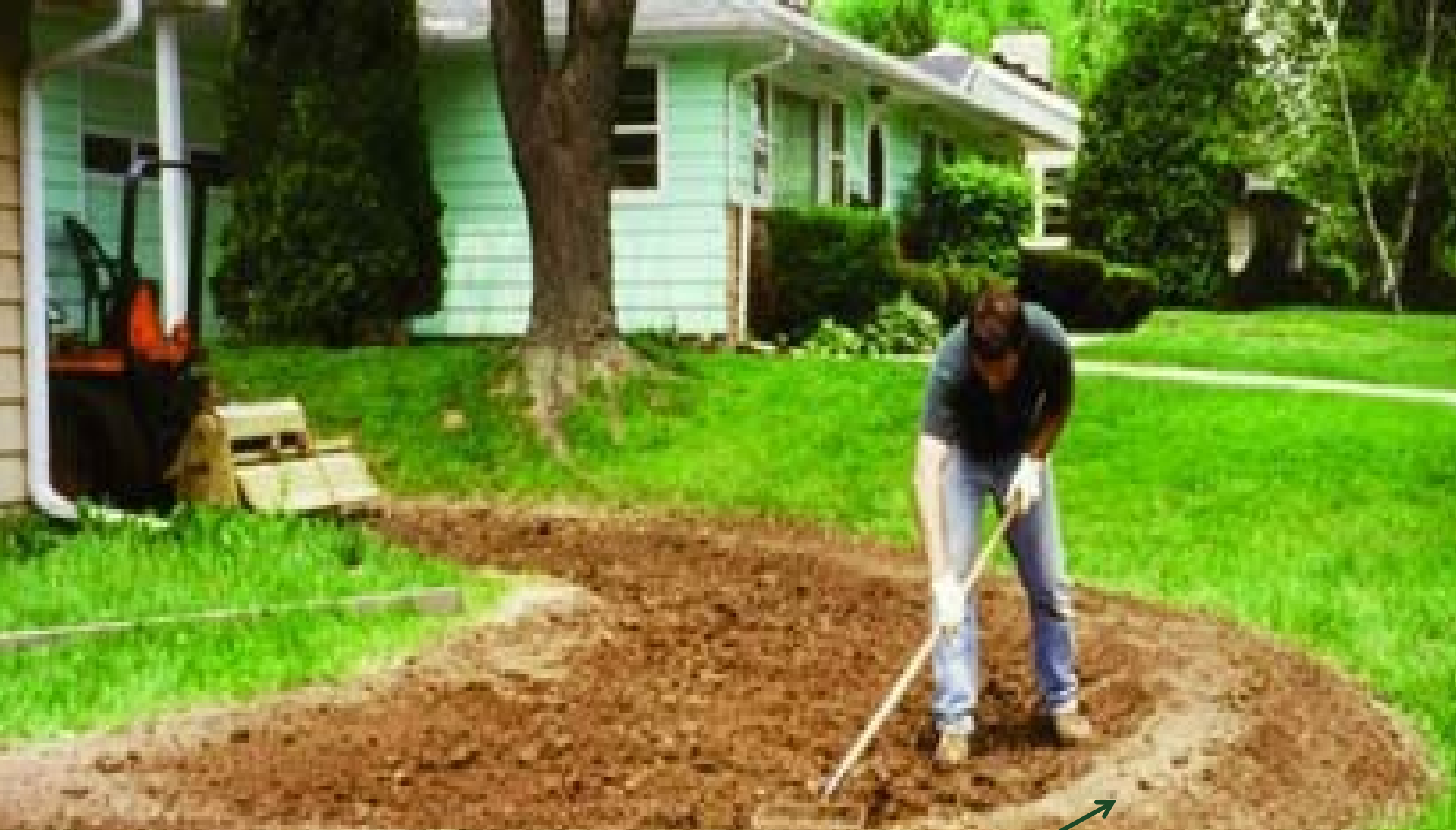
After digging out the area, build berm on downhill side of the rain garden. Level the garden's base and prepare for planting.
